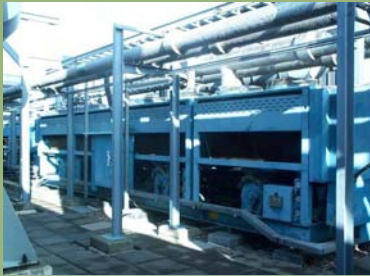
Ware R&D Building 5 Chillers
